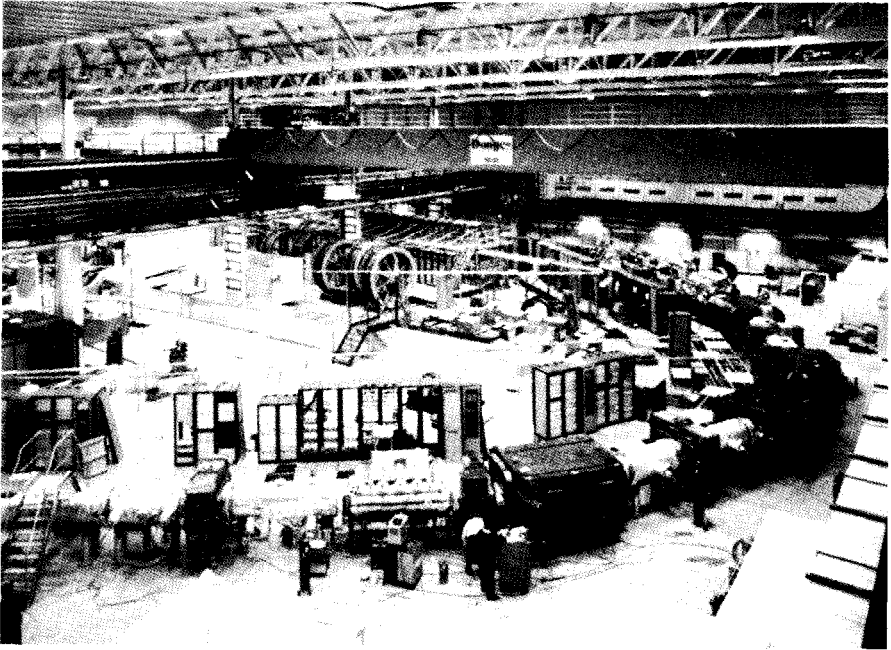
Fig. 15. View of the Antiproton Accumulator before it was covered by concrete slabs. The silvered material around the vacuum tanks is insulation, needed because everything may be heated to 300° to obtain ultra-high vacuum. The transmission lines crossing the ring and carrying the cooling signals may be seen.
